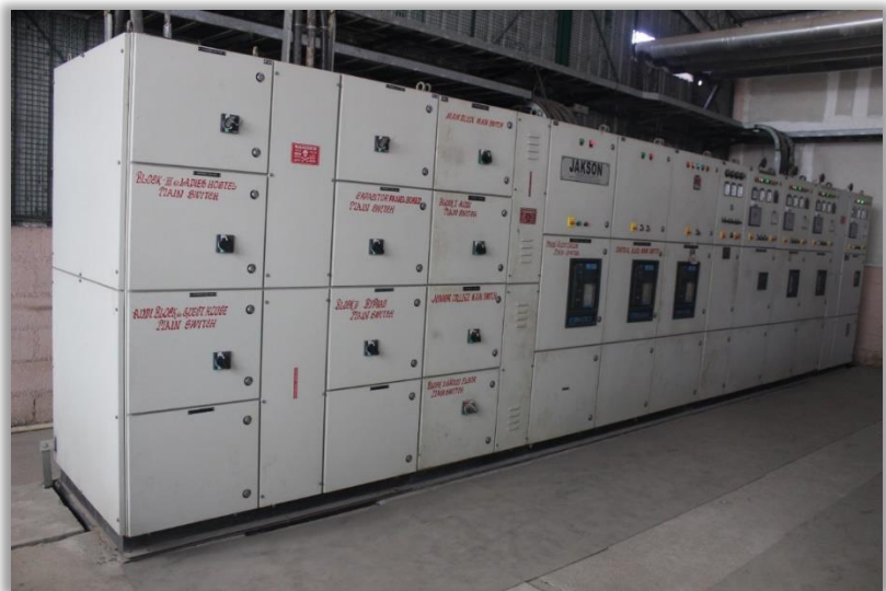
Figure 1. Main control panel
