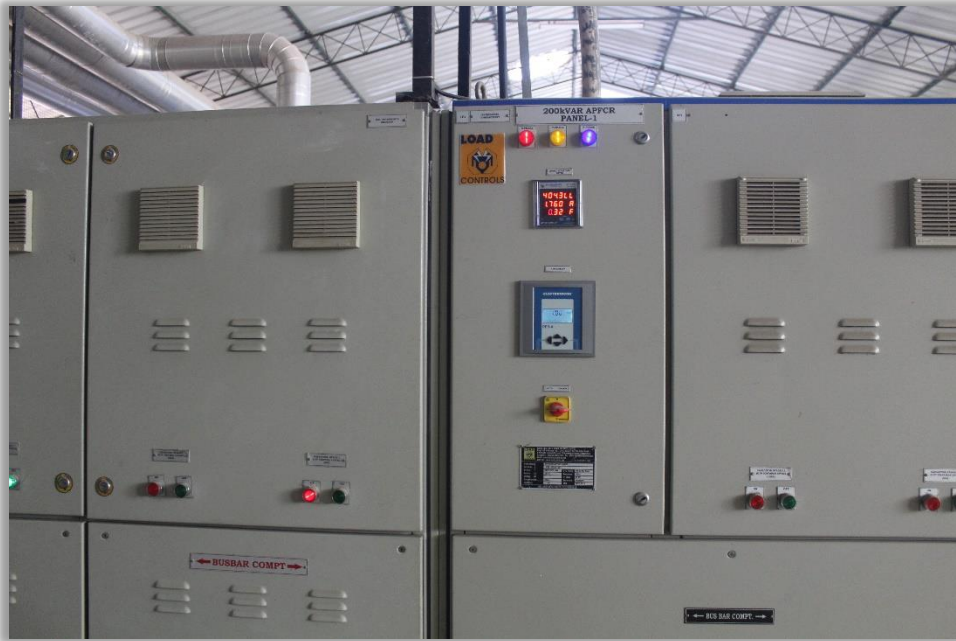
Figure 3. Capacitor bank (APFC)
