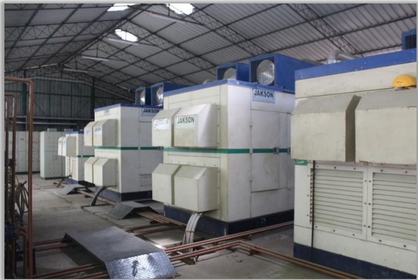
Figure 2. DG Sets at control room
